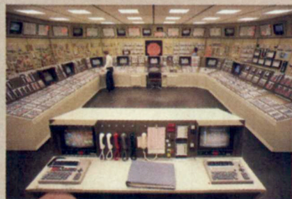
Hope Creek power plant control room simulator.
